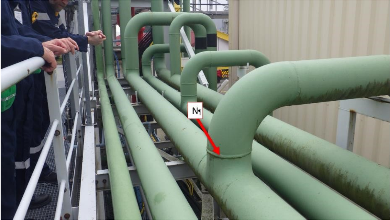
Figure 12 Shows large T-section and Elbow used (delineated by N) to test UT Crawler.
