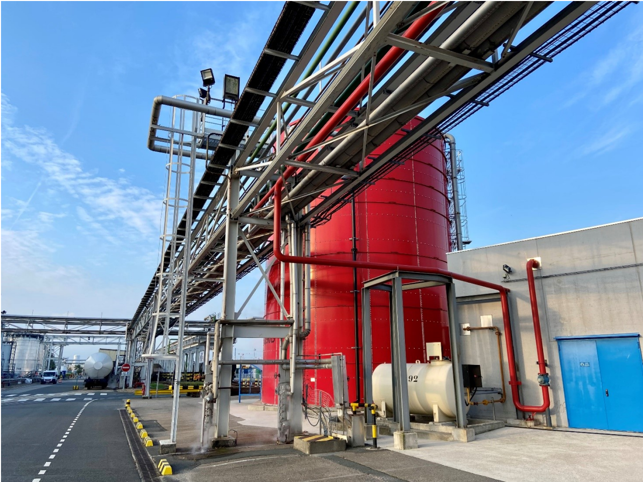
Figure 3. A detailed view of the Chevron Oronite plant with a pipe rack.
