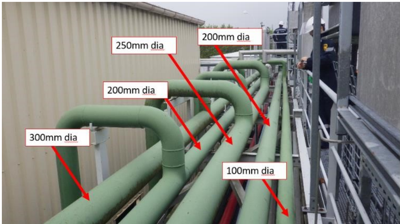
Figure 10 Showing raised pipe rack with piping diameter. Testing was conducted on the 250mm Diameter piping (8 inch).
