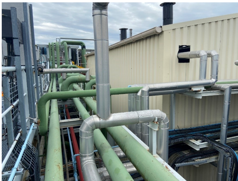
Figure 2. A detailed view of the Chevron Oronite plant with piping.
